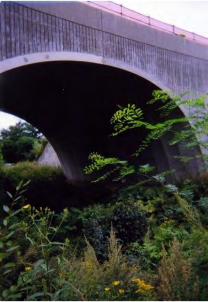
Figure 2. An arch type culvert over the natural habitat of Cambaroides japonicus and their endemic branchiobdellids in Hokkaido, Japan.
